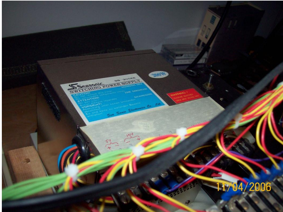
VIEW OF POWER SUPPLY BEHIND AGUA LA SAL PANEL
